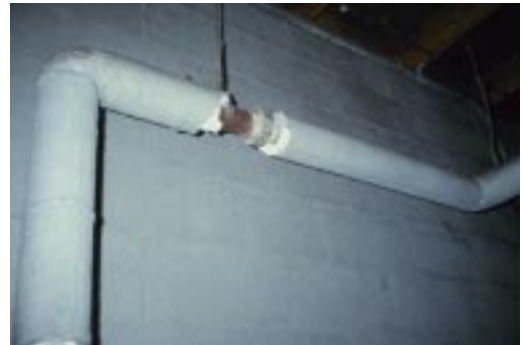
Asbestos insulation on a water pipe.
